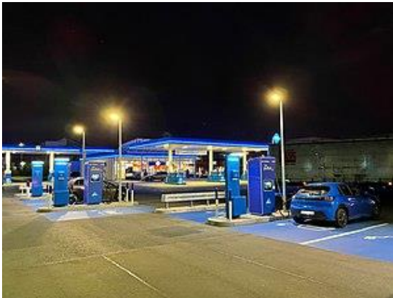
Aral Pulse charging stations in front of a Aral -branded BP gas station in Braunschweig , Germany
